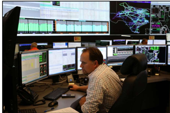
ERCOT Manages the Flow of Power Supply in Texas
